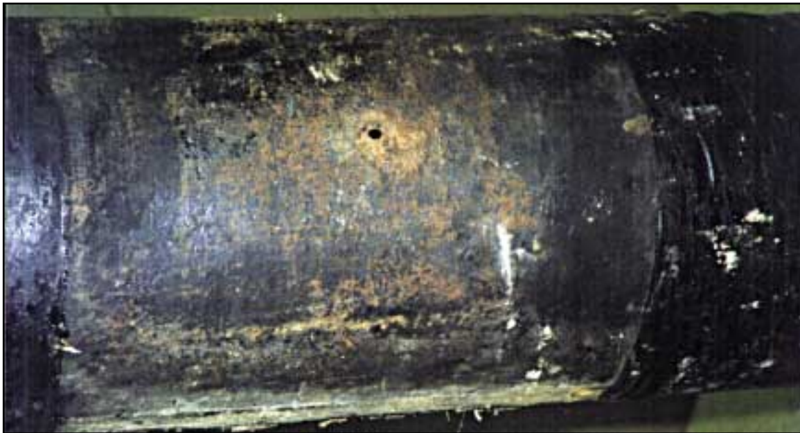
One of a family of pits originating along the pipe interior that penetrated the pipe wall.
