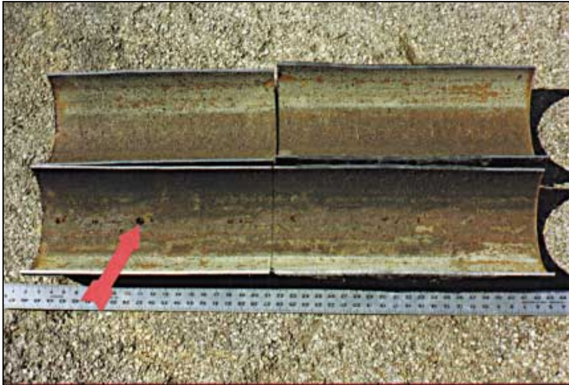
Cross section of pipe showing location of pit
