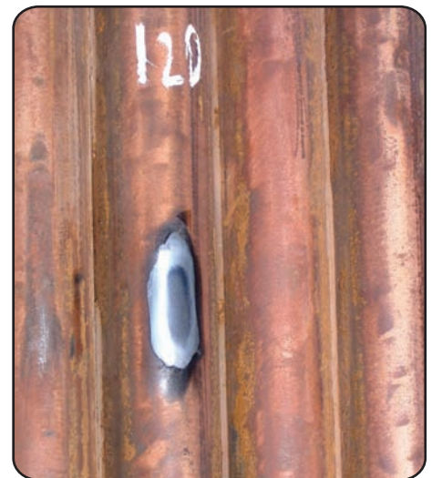
Polished FMR site on a boiler tube
