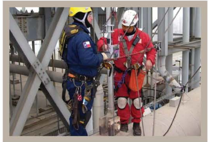
Installation of Pipe Hanger Load Monitor
