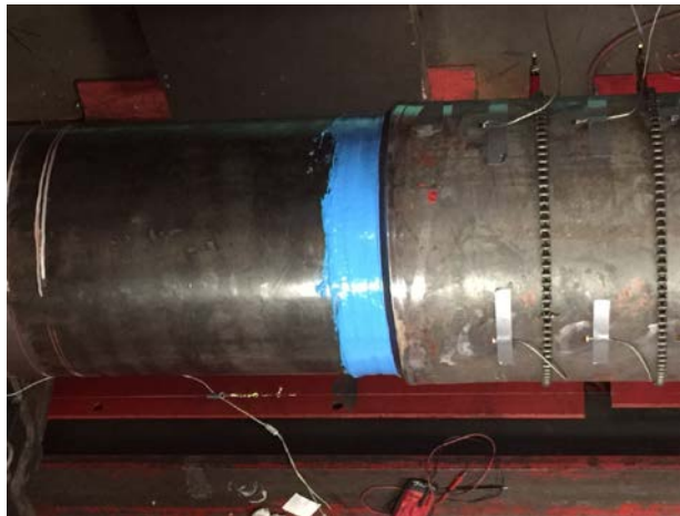
Figure 4. Joining operations for Sample 1 (406-mm OD x 21.4-mm Wall Thickness, Grade X52 (Actual Yield Strength of 71.5 ksi)).
