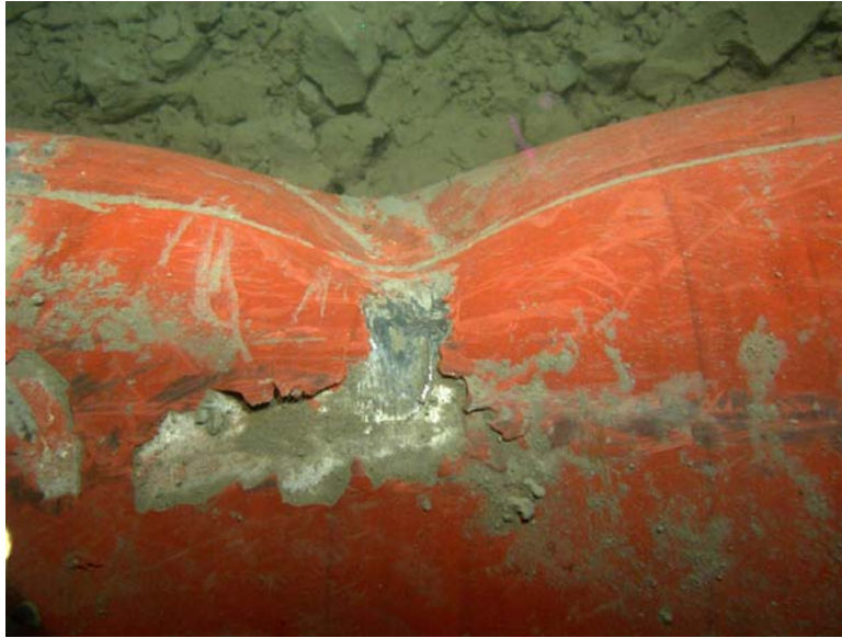
Figure 5 – Photograph of dent in 20-inch Shell URSA gas pipeline [15]
