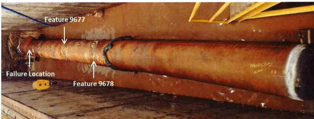
Figure 16: Photograph of Sample 4 after burst test sample. Failure location and several flaws identified by ILI are labeled.
