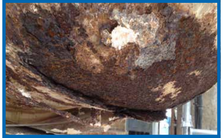
Corroded vessel: Corrosion Under Insulation (CUI)
